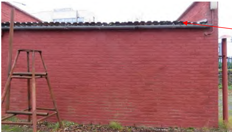
Photo 27 – potential roosting sites under roof
